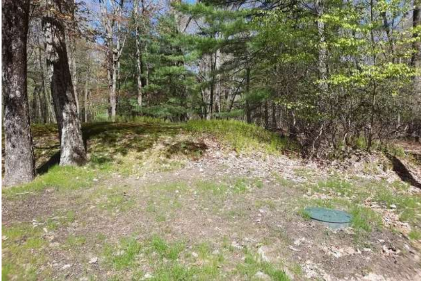
This wastewater system consists of a sand mound for effluent absorption with a septic tank in the foreground where you can see the access panel. Photo: Peter Wulffhorst, Penn State
