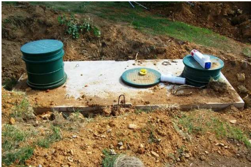
Homeowners should make a map showing the location of the components on their on-lot septic system. Photo: G. Hurd, Penn State Extension
